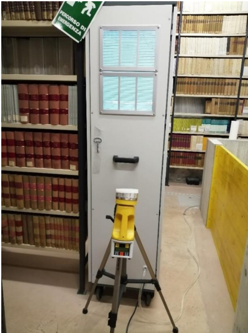
Image 2: Air Treatment Device
